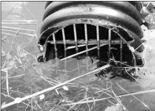
Outfall # 4 located by an open area of turf grass drains directly into the Scugog River.
