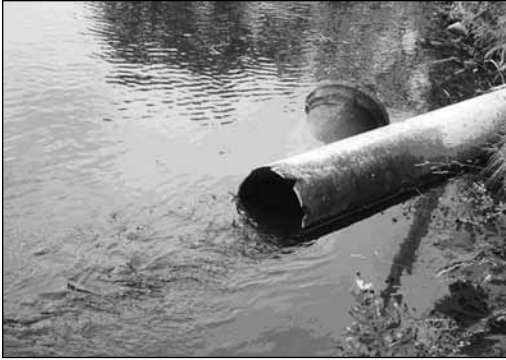
Outfall # 2 at the end of a residential street drains directly into the Scugog River.
