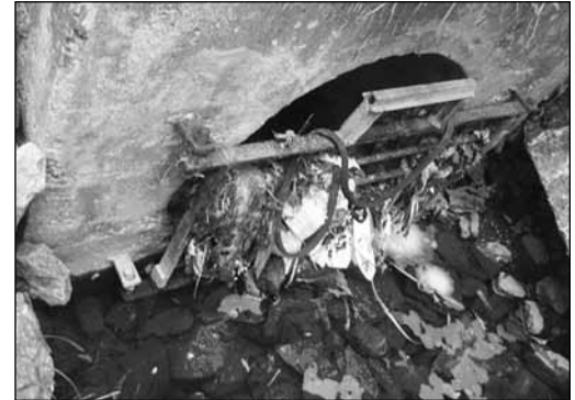
Outfall # 3 on the east side of the river flows through a channel to drain into the Scugog.
