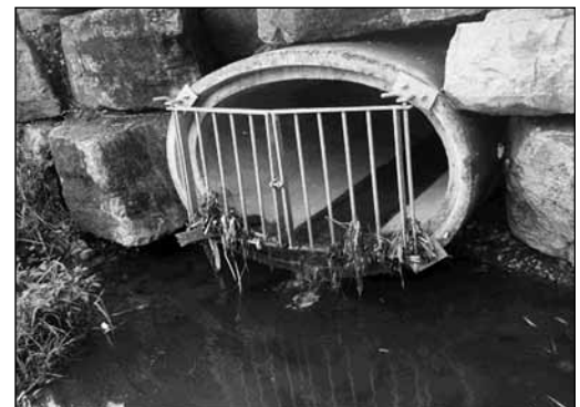
Outfall # 5, very close to Kent Street, drains into a holding area that leads to the river.
