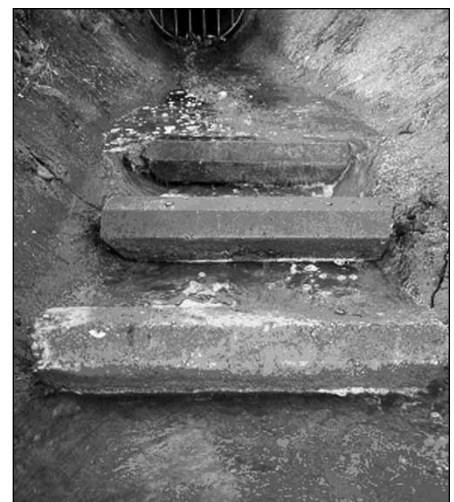
Outfall # 7, located near the city core, has cement blocks to alter the flow leading to the Scugog River.
