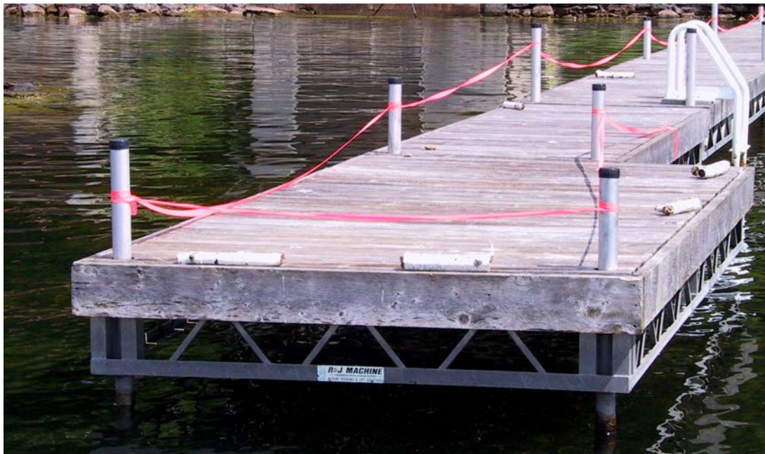
Bird proofing dock
