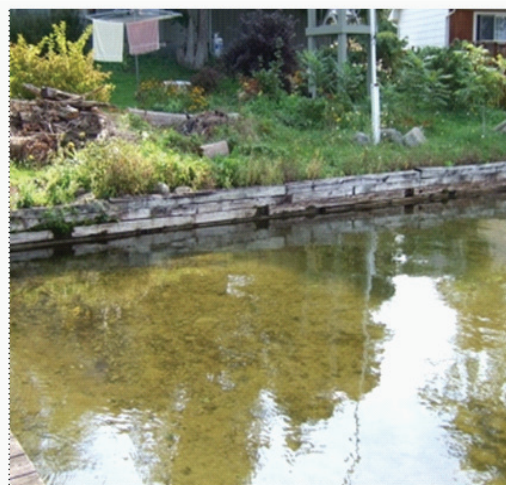
Fig. 2 (Before): Wooden structure holds the soil in place. Photo by Kawartha Conservation
